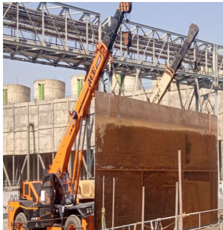
80 MT crane was deployed to lower the C section into the channel.
