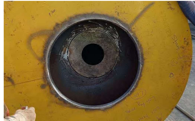
5. Similarly center marking & cutting of inner diaphragm was done to fit plate 2A.
