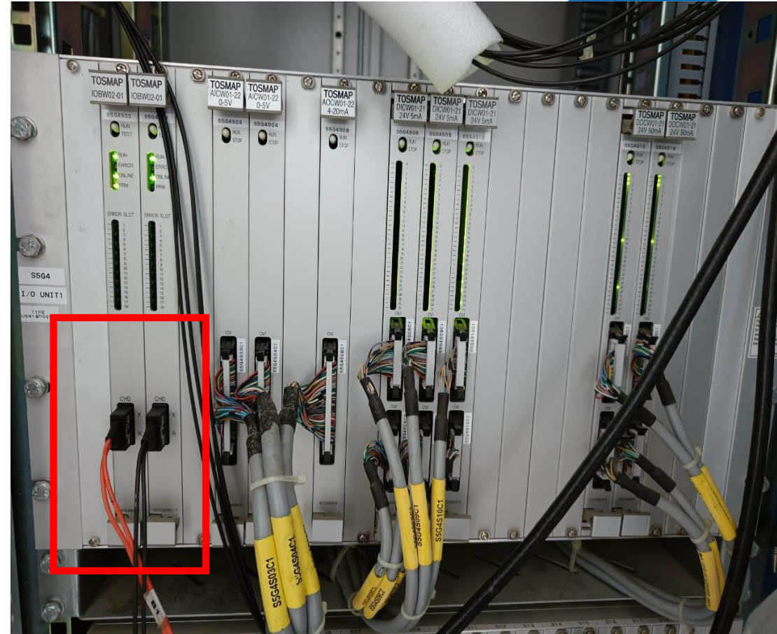
CPP RIO PANEL UNIT-1/UNIT-2
