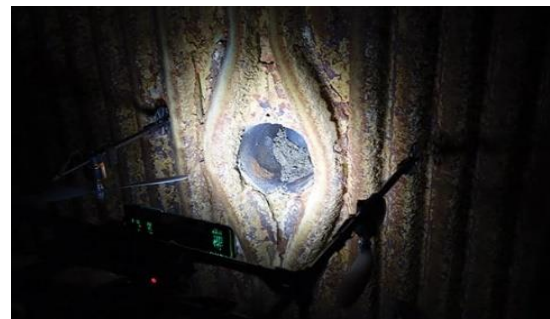
Wall blower opening area inspection by Magnetobot drone
