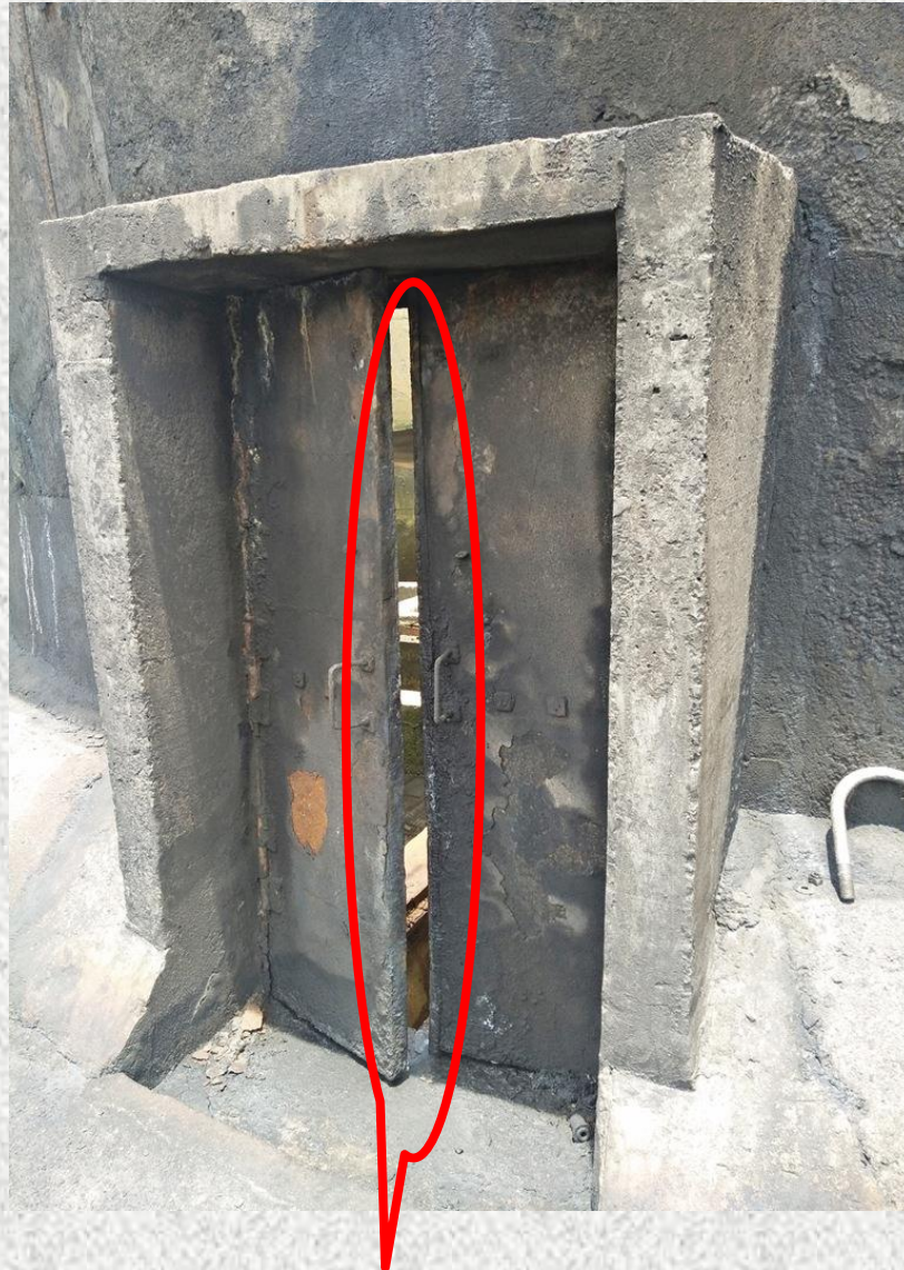
Poor workmanship in fixing the access door
