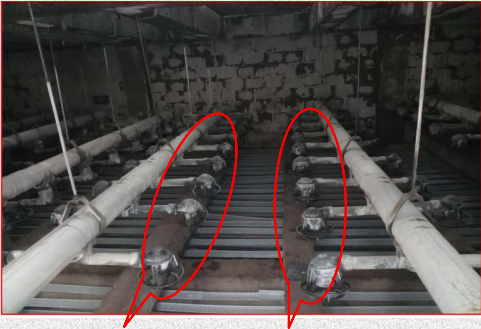
Complete Fouling of Nozzles with Support Beam
