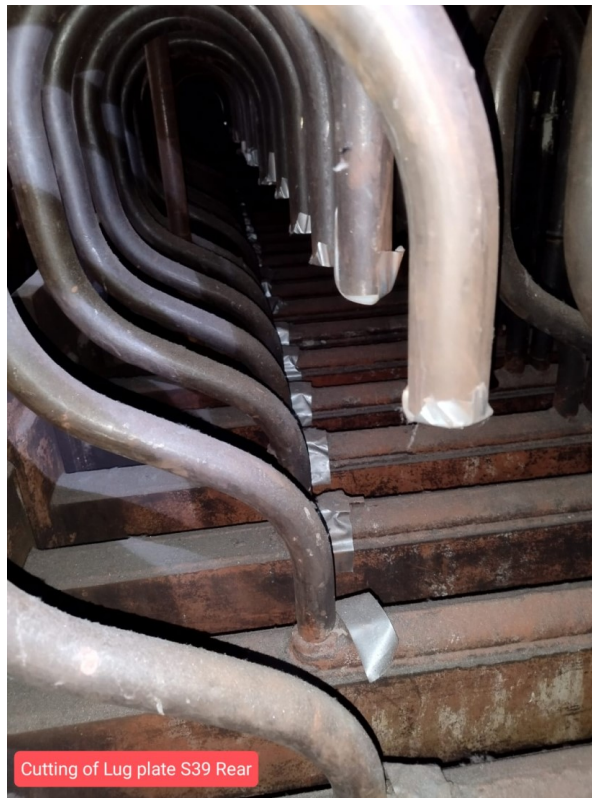
Covering of cut tubes with tapes to prevent ingress of foreign material
