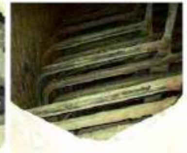
After an on-line cleaning
