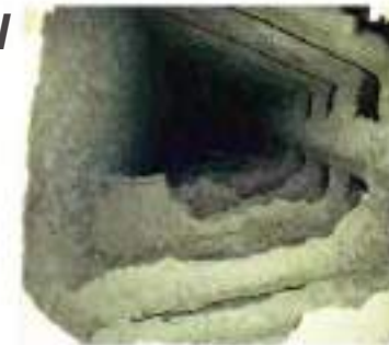
Before an on-line cleaning
