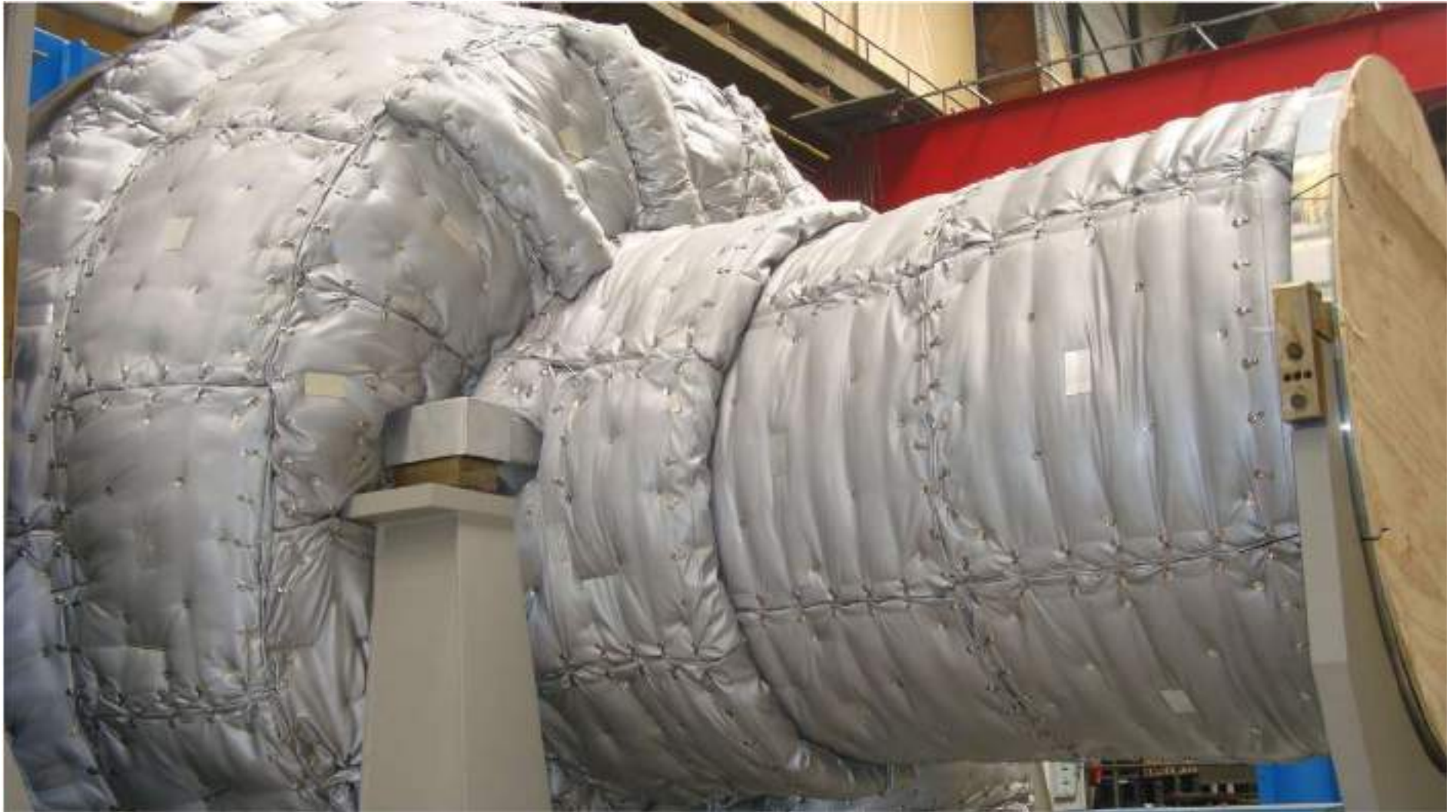
Pillow noise insulation on gas expander
