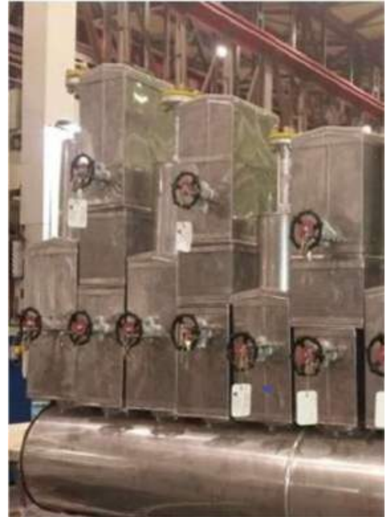
Sheet metal jacketing control panel
