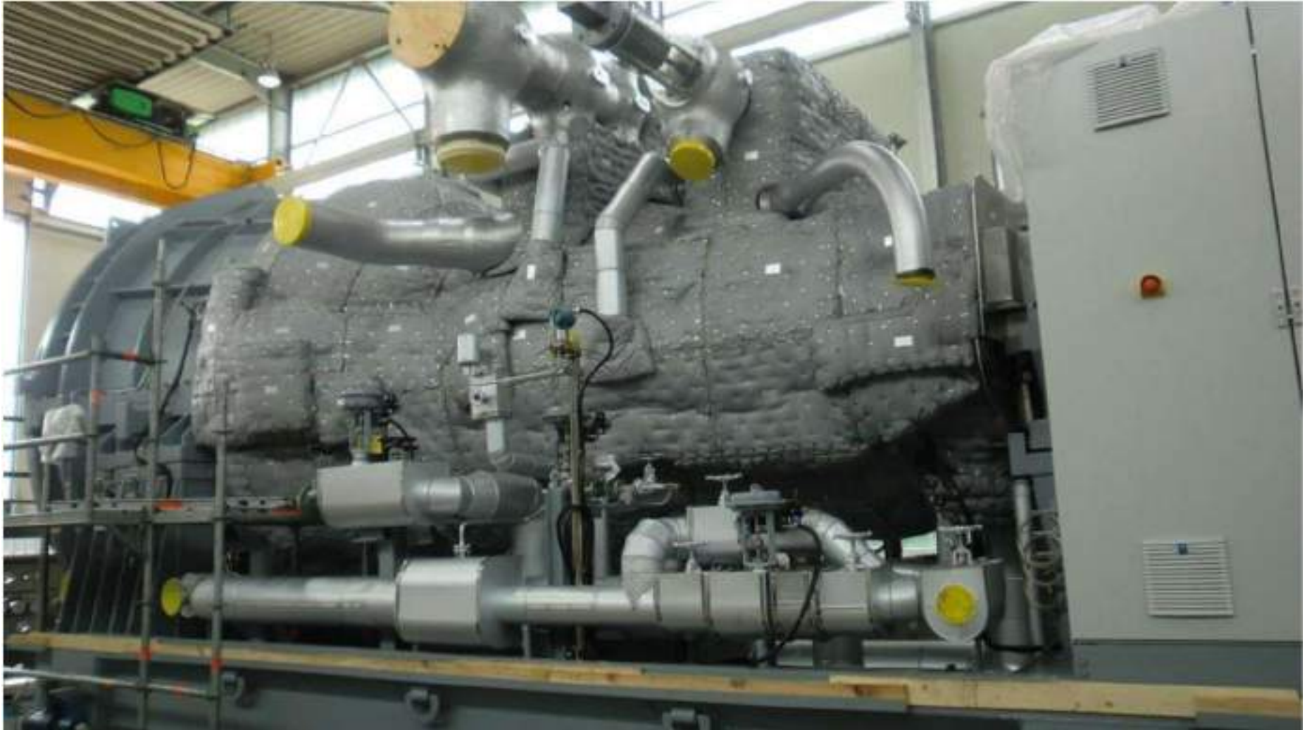
Pillow insulation (flat shape) on steam turbine
