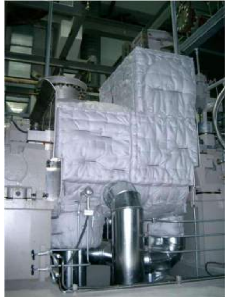
Pillow insulation with sandwich heat retention shield on industrial steam turbine
