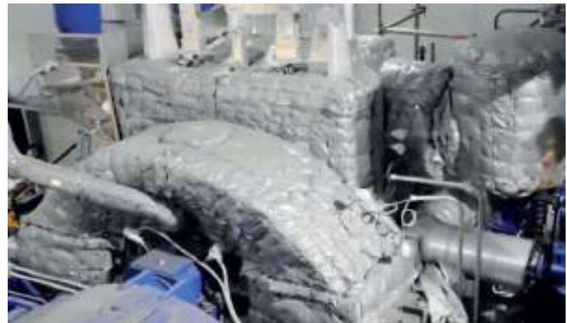
Pillow insulation (flat shape) on steam turbine
