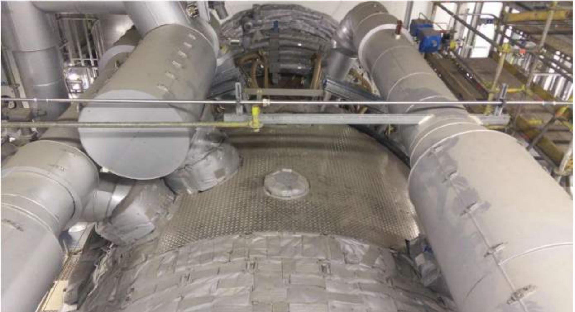
Pillow insulation (spherical shape) on gas turbine
