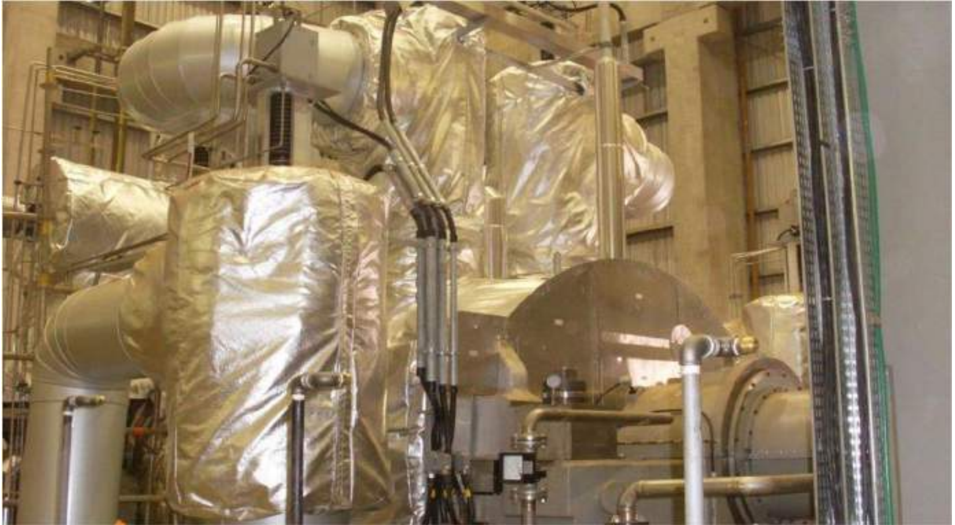
Glass fiber cover on steam turbine
