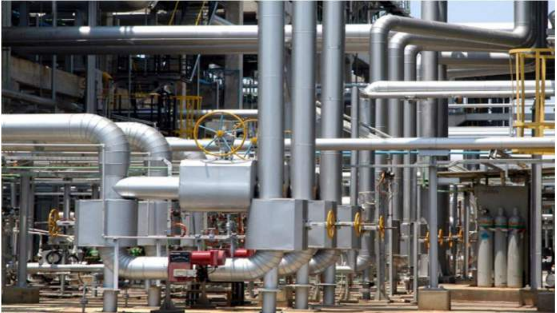
Sheet metal jacketing on insulated outdoor piping of petrochemical facility
