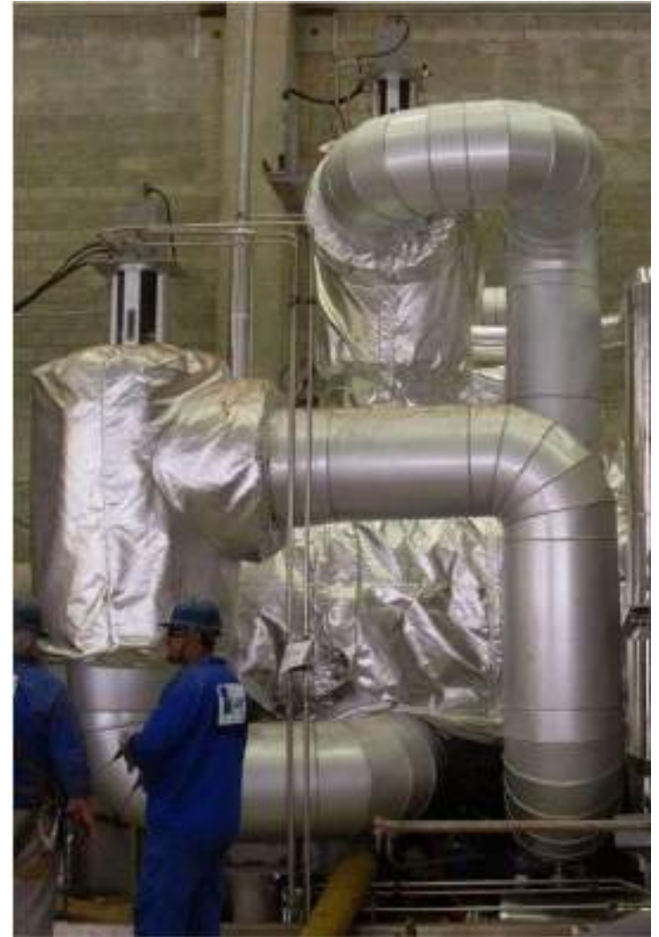
Glass fiber cover on steam turbine
