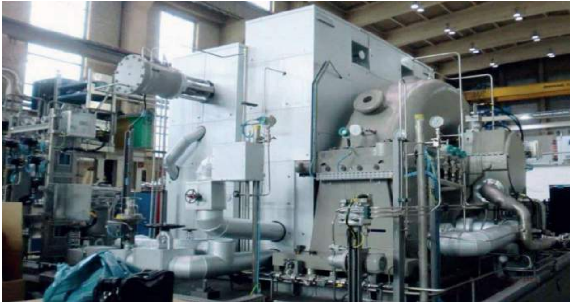
Enclosure on industrial steam turbine
