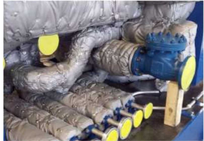
Pillow insulation (spherical shape) on steam turbine piping
